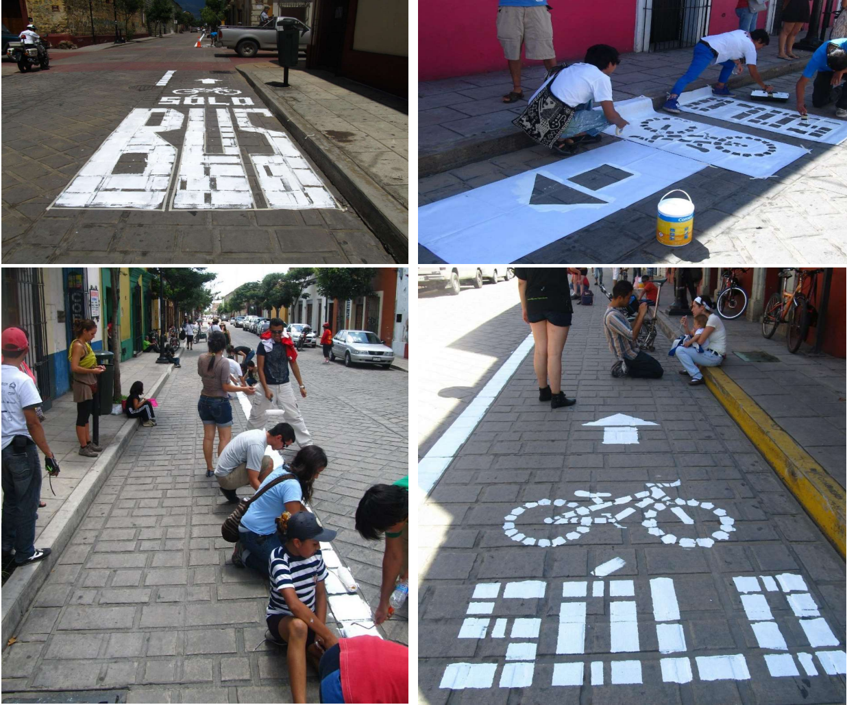
Figure 10. Citizen cycling lane during 2012 Bicired National Cycling Conference (photos by Claudina de Gyves)
